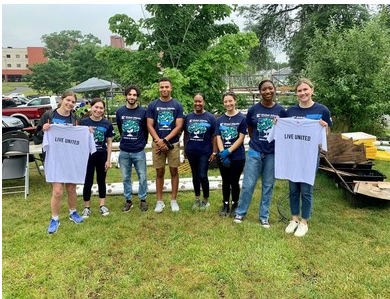
Global Atlantic Financial Group Interns installed hydroponic garden structures at Levo International.
